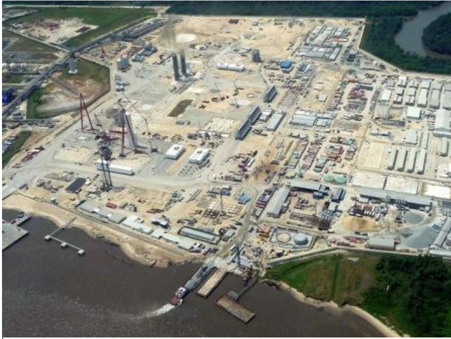
Construction at the Escravos LNG terminal; the sector, and infrastructure development in it, is a huge boost for the protective paints industry.
